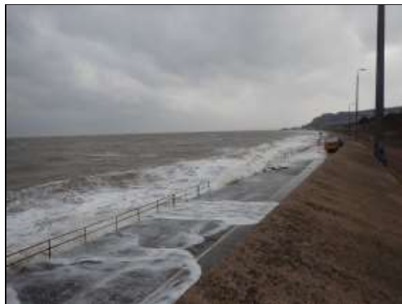
Damage to railings
