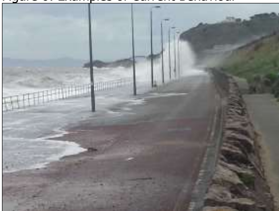
Typical overtopping on spring tide (March 2013)
