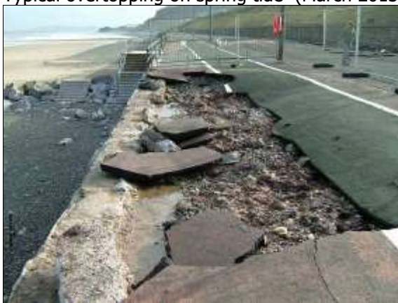
Damage to promenade surfacing
