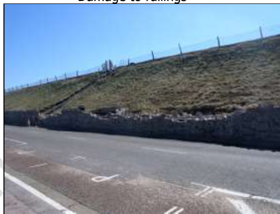
Damage to NR boundary wall and embankment
