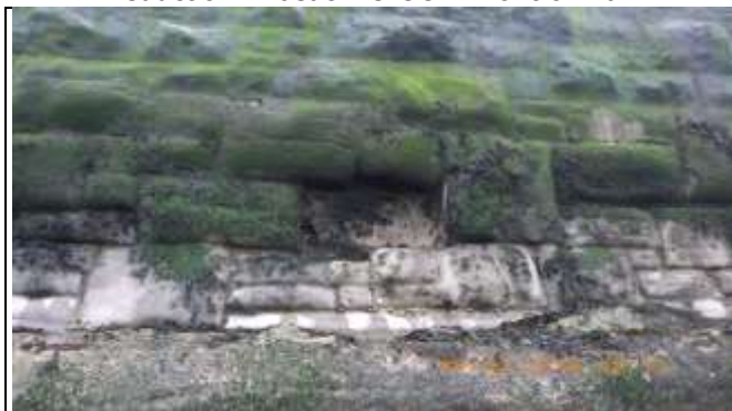
Loss of Blocks to Sea Wall
