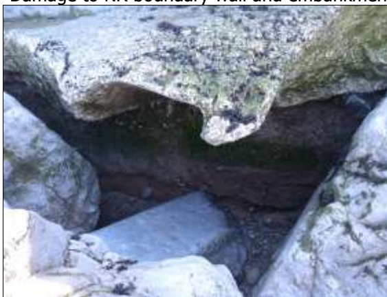
Sea Wall Undermining
